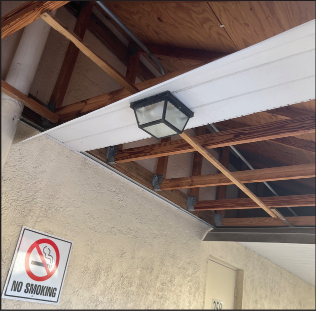
Several roof panels from an office in Venice are nowhere to be found following the hurricane. Businesses and homes alike suffered property damages due to intense wind gusts. PHOTO BY KAI SPRUNGER
