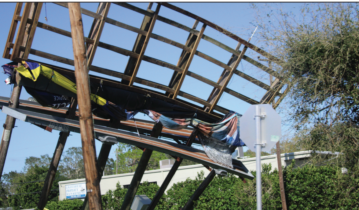
A fallen billboard leans on the side of Highway 41 on a route back to Sarasota from West Palm Beach. Ninth-grader Ava Lernerz and her family evacuated to the eastern Florida coast as Hurricane Ian's path veered toward the Sarasota area. PHOTO BY AVA LENERZ
