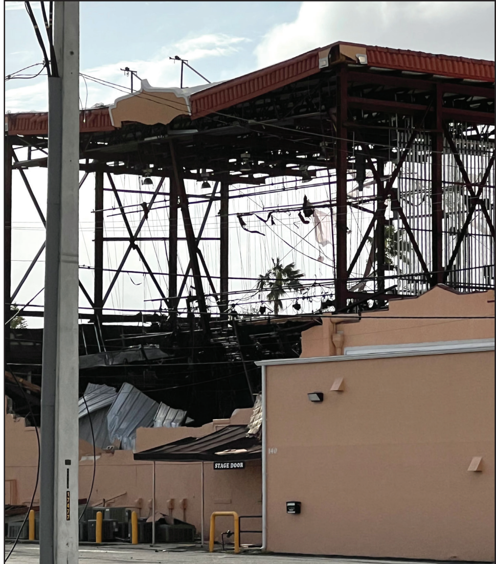
Venice Theatre barely stands following the intensity of the hurricane. Restorations to the theater's main stage house have already begun but are projected to take over eight months. PHOTO BY KAI SPRUNGER
