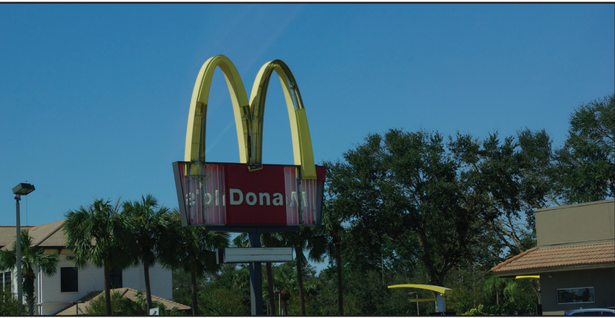
A McDonald's sign stands upright following the storm, but not without its fair share of damage. Many businesses had to make quick repairs to their exteriors prior to reopening. PHOTO BY ALYSON MIZANIN
